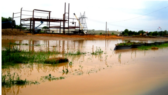
Runoff from a construction site after a recent rain event overwhelms the silt fence and other BMPs, leading to major flooding of the roadway and sediment entering the storm drains.
