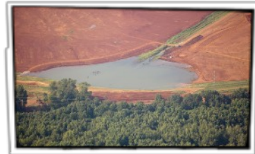
“This photo, depicting early progress on stormwater-control measures for the site, was taken by SouthWings during surveillance in August 2018.”. Flight by SouthWings.org
