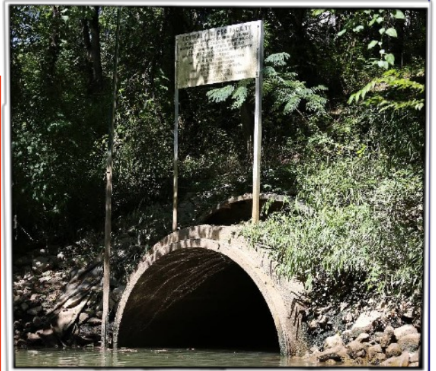
Sewage pipe in Chattanooga, Tennessee.
